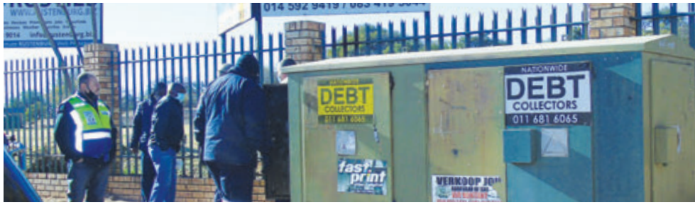
The victim's body was trapped inside the high-voltage mini substation.
